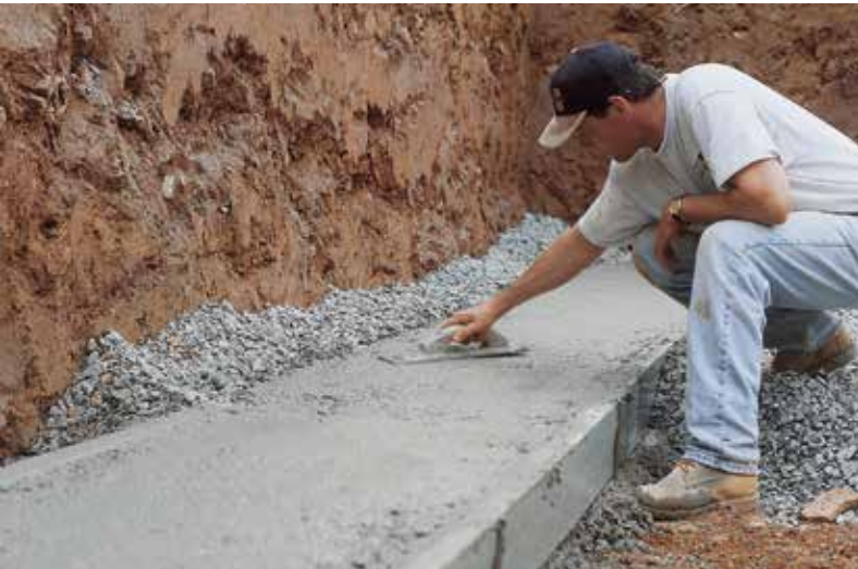
During the concrete pour, grade stakes hold the Form-A-Drain Plus system at the proper elevation. Thereafter, Form-A-Drain Plus remains permanently in place.
